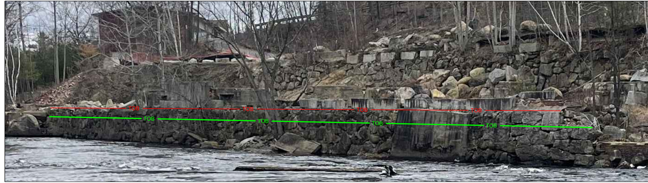
LOOKING AT THE SITE RIVERSIDE RETAINING WALL, WITH LINES DEPICTING THE EXISTING TOP (RED) AND PROPOSED TOP (GREEN). THESE LINES ARE APPROXIMATE; THE EXISTING TYPICAL WALL TOP ELEVATION IS 576.2' AND THE PROPOSED FLOODPLAIN ELEVATION AT THE WALL IS 574.0'.
