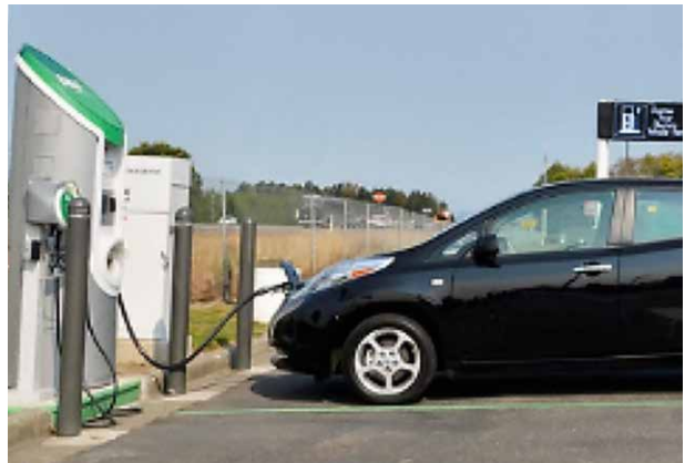
Figure 2.1. Level 2 chargers (top) are common in home, workplace, and public settings and can charge a BEV from empty in 4-10 hours. Direct-current fast chargers (DCFC) (bottom) are common as public chargers and along highway corridors, and can charge a BEV to 80 percent in under an hour. (Photos: ©123rf.com/ flippo [top]; Washington State Dept of Transportation [bottom])
