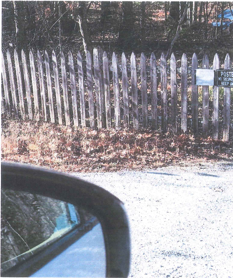
A fresh coat of a suitable color would transform this fence from unacceptable to acceptable.
